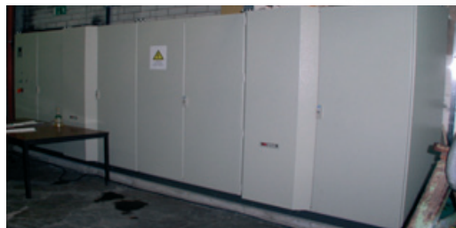
Control cabinet new
