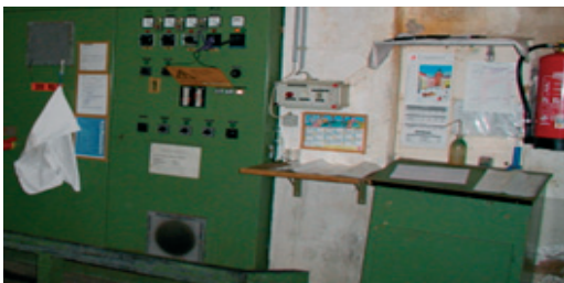
Control cabinet old
